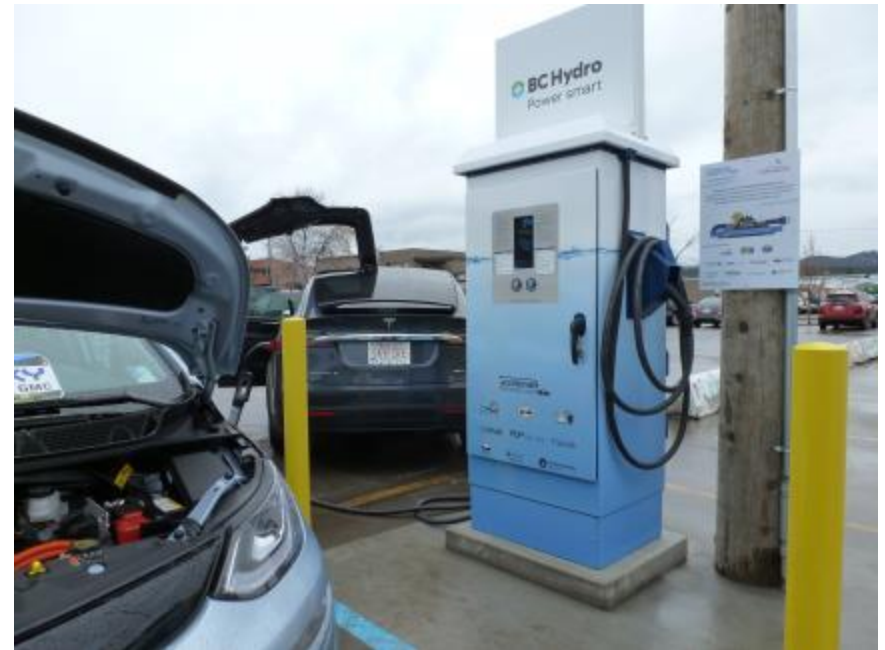
DC fast charger in Cranbrook, B.C.
