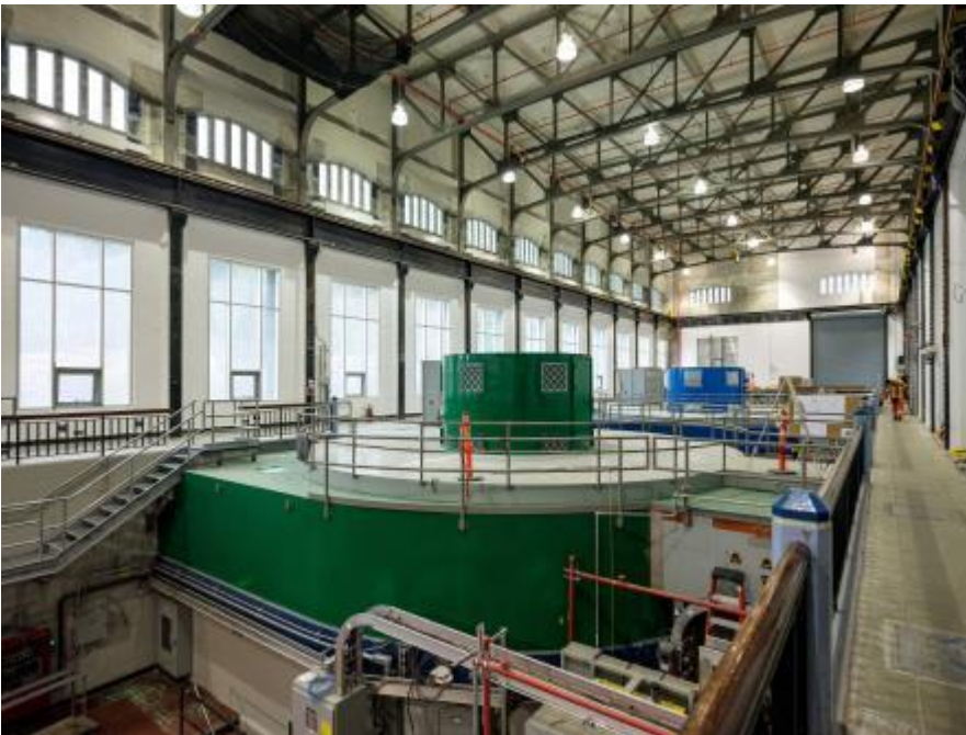
Ruskin Dam generators
